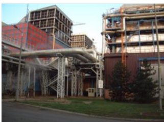
GT1 + CST17 CCGT 205 MW, 1991 -
