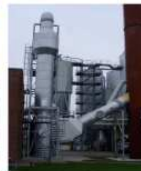
Alstom Flue Gas Condenser
